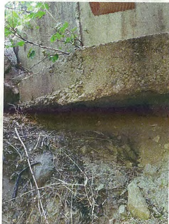
Photo 22 – Severe Scour at East Abutment
