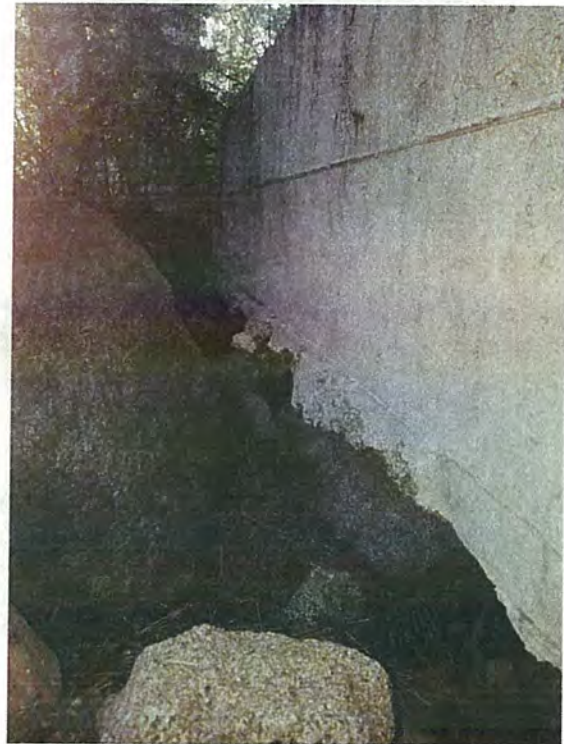
Photo 4 – Scour at West Abutment Footing
