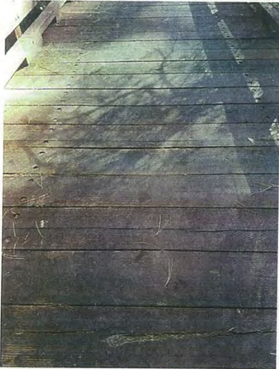
Photo 19 – Wearing at Deck Surface
