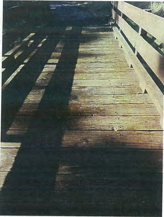
Photo 27 – Moderate Wearing at Deck Surface
