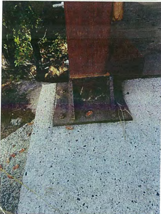
Photo 21 – Missing Bolt at End Post Connection
