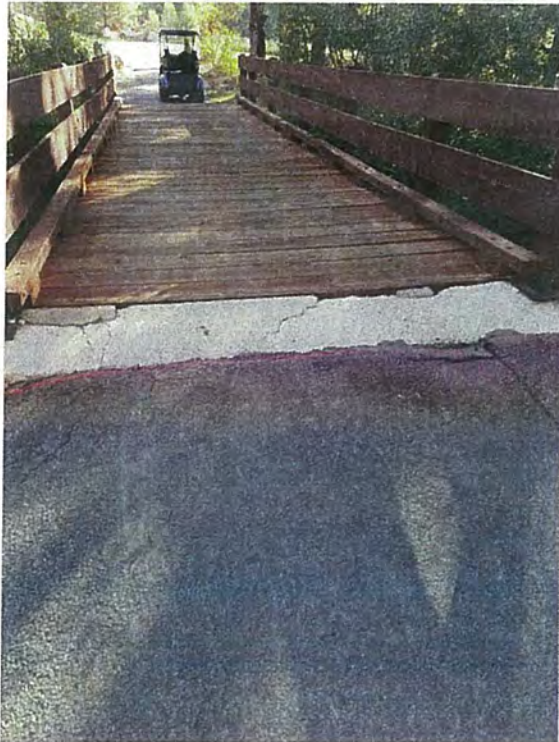
Photo 7 – Cracking and Spalling at West Abutment Approach Apron
