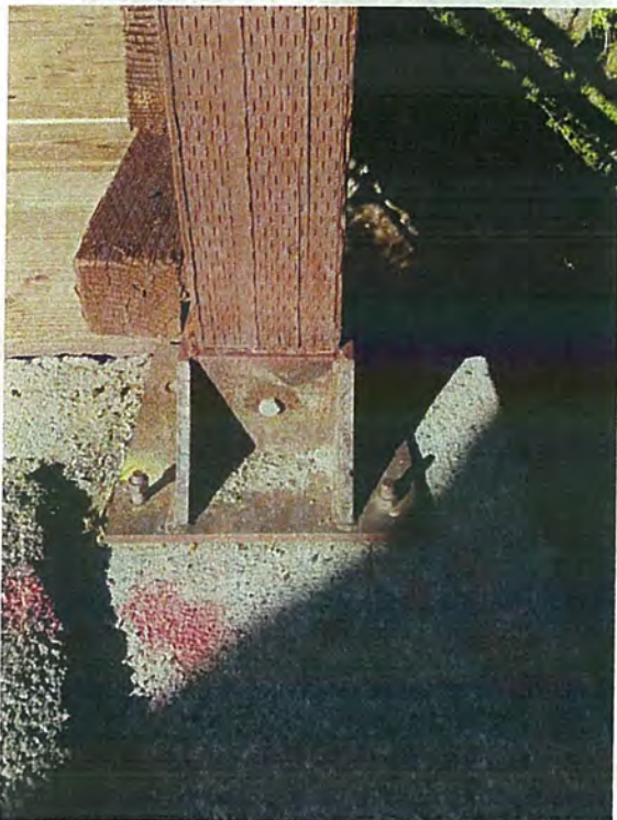
Photo 11 – Slight Corrosion/Missing Anchor Bolt
