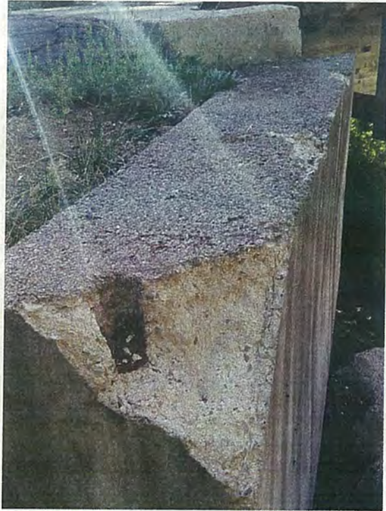
Photo 24 – Spalling at Northwest Wing Wall
