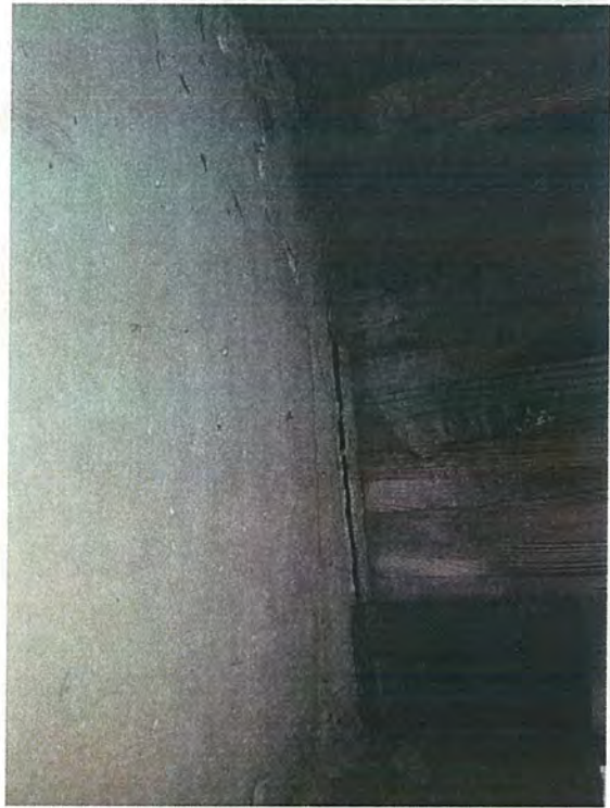
Photo 14 – Spalling at Top Connection at South End Beam Bearing
