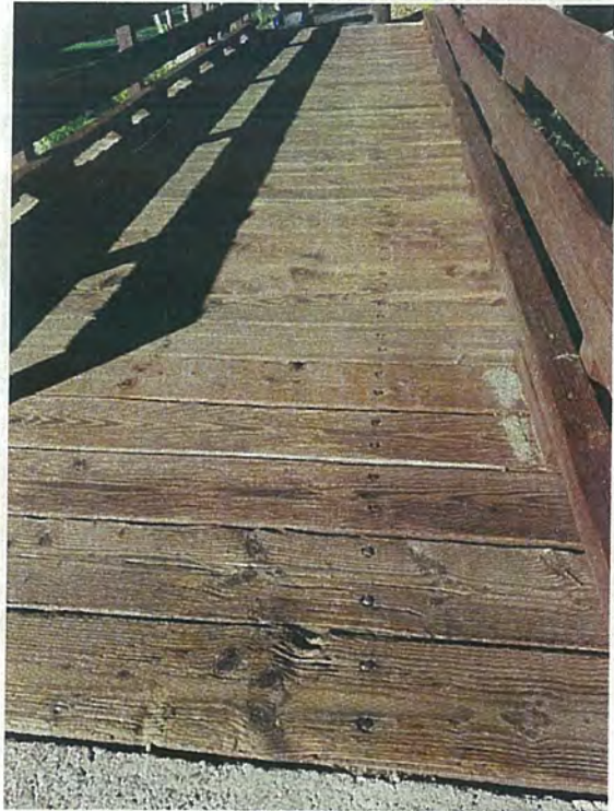
Photo 10 – Wearing at Deck Surface
