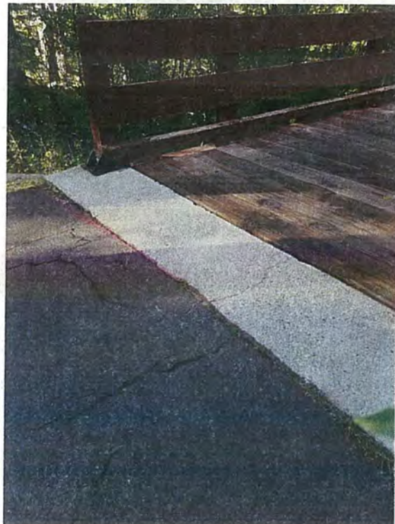
Photo 8 – Crack at East Abutment Approach Apron
