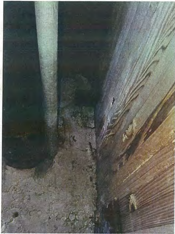
Photo 6 – Spalling at Top Connection Southwest Beam Bearing
