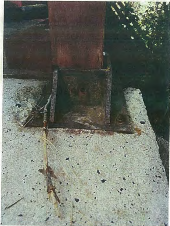
Photo 20 – Missing Bolt at End Post Connection
