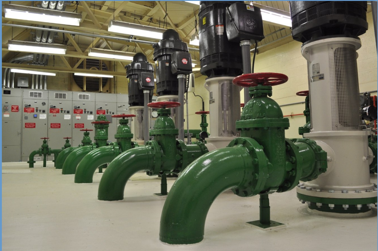
Spoooner Pump Station
