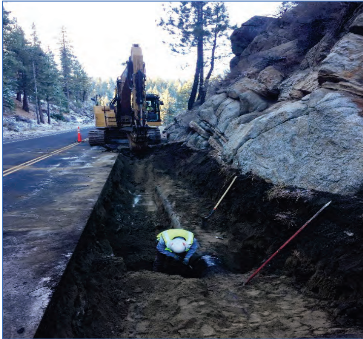
Figure 4. Example of open trench excavation and pipeline installation adjacent to highway in Lake Tahoe Basin.
